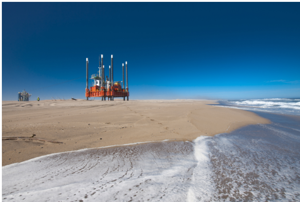
The sea walker drill platform is drilling the surf zone for grade control. The platform is accessible via an aerial ropeway and is the first stage in the development of a larger drill platform.
